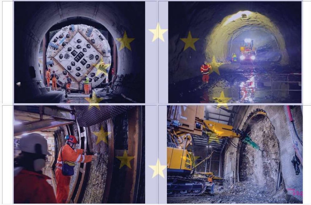
Works for the construction of the base tunnel of the Mont Cenis
